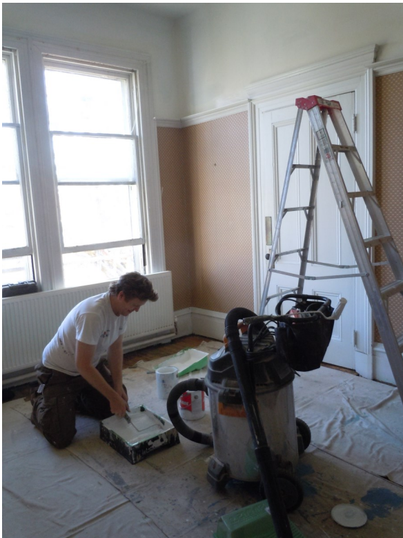
Painter putting the last coat of paint on newly repaired ceiling and walls.
